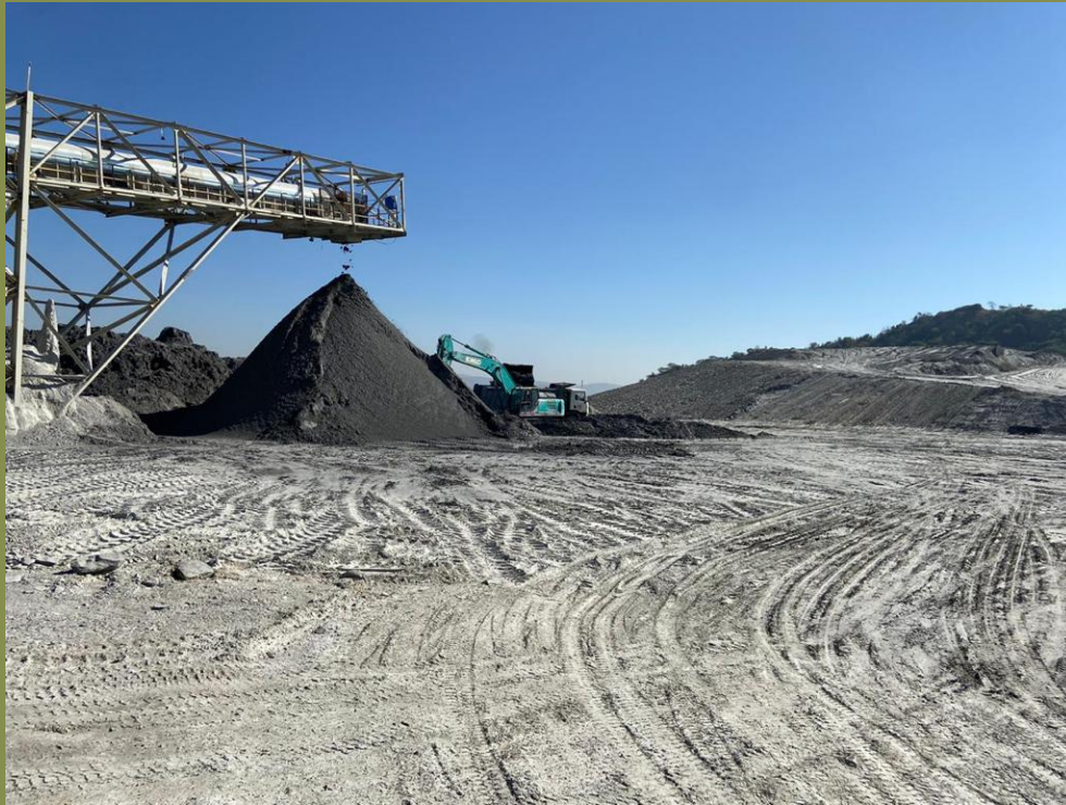
The worksite of the tailings dam expansions. Photo credit: Dhaatri Resource Centre for Women and Children
