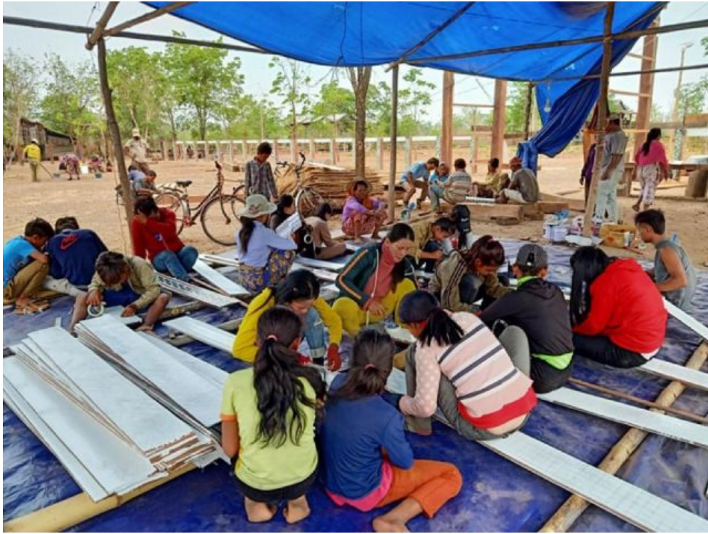
Construction of cultural centre by the Kbal Romeas community during lockdown. Source: CIWWG
